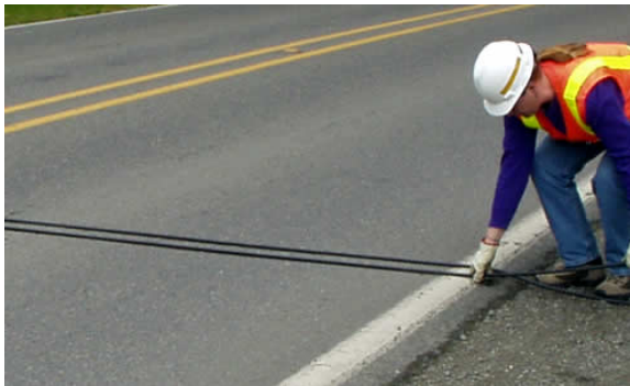
The installation of road tubes on a roadway
