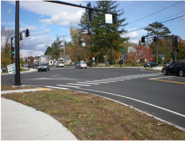
Pedestrian improvements completed at the intersection of Silver and Federal Streets in Greenfield
